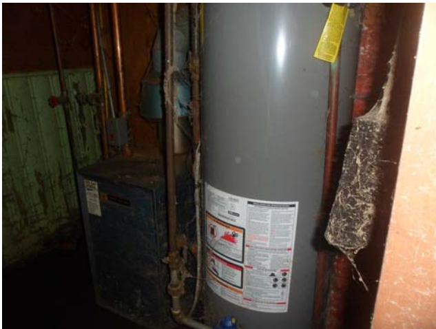
#9: View of the boiler located in the basement.
